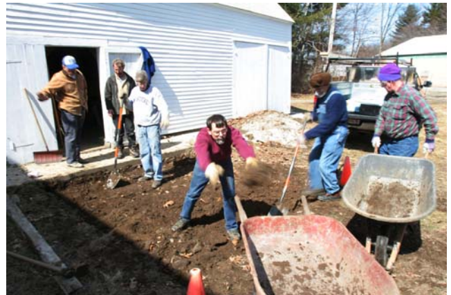
Removing soil for the cement platform. (L-R) Paul Cicchetti, Dave Prowten, Steve Clougherty, Mike Hill, Bill Toomey and Dave Wilber
